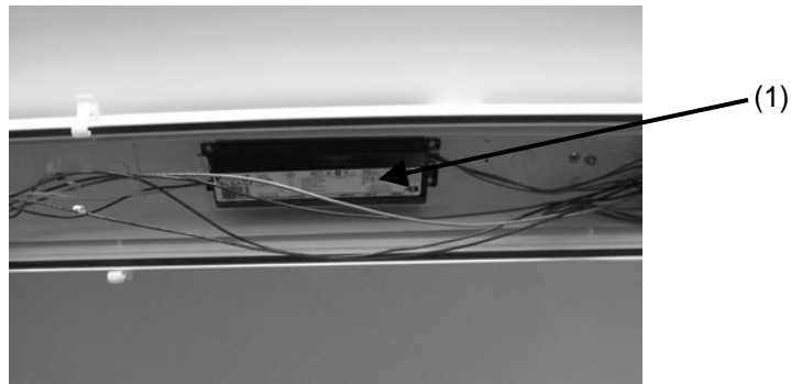
Figure 4-43. Ballast in ceiling light fixture.
