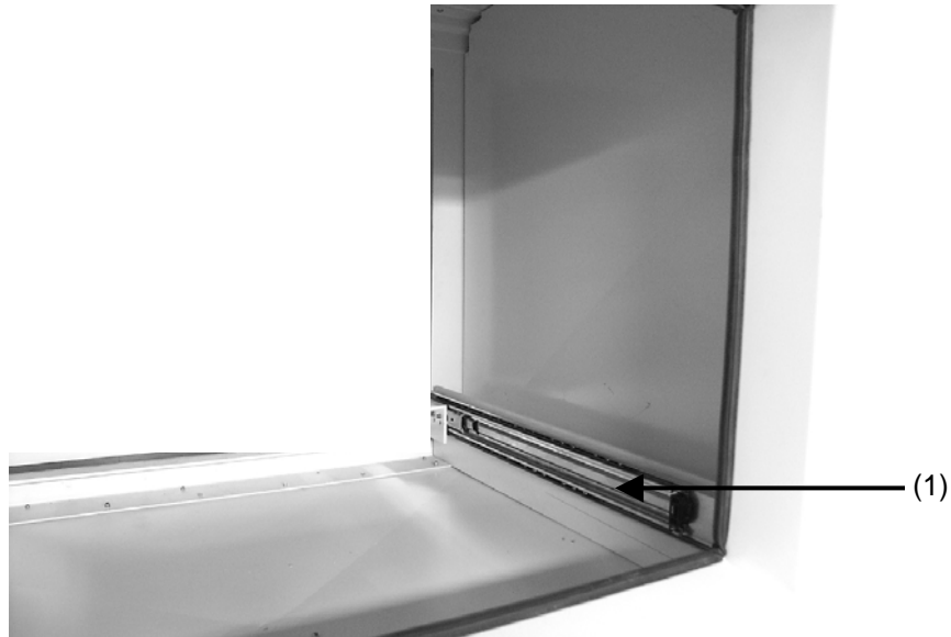
Figure 4-23. View of ECU compartment from inside container.
