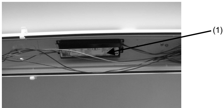
Figure 4-8. Ballast in light fixture.
